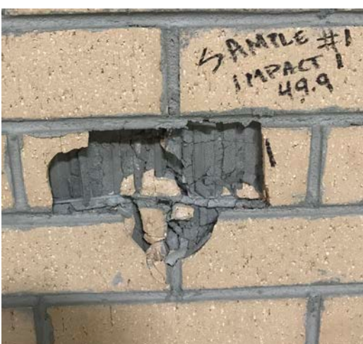
Figure 1- Impact location #1 front view
