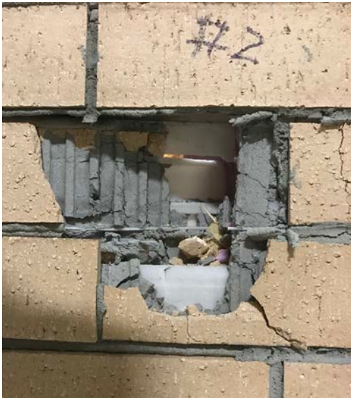
Figure 3- Impact location #2 front view
